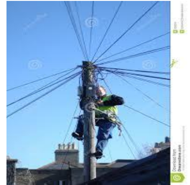
Telephone Drop Points (DPs) (Still in Use in Urban Areas)
